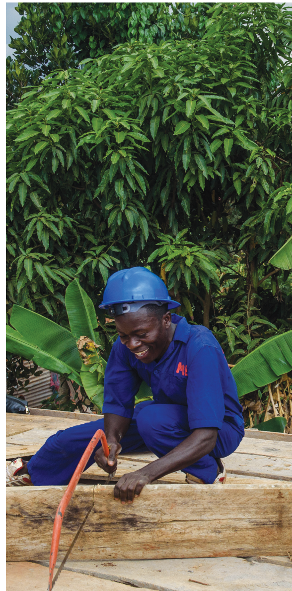
U-LEARN II TRAINEES RECEIVE HANDS-ON TRAINING AS THEY BUILD A NEW HOSTEL IN UGANDA.
